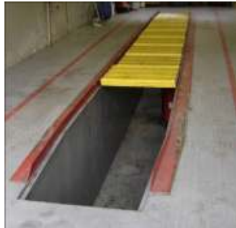
Swain Co. has installed OSHA approved safety grate
